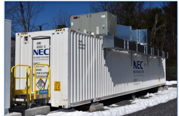
Sterling, MA 2 MW / 3.9MWh Energy Storage
